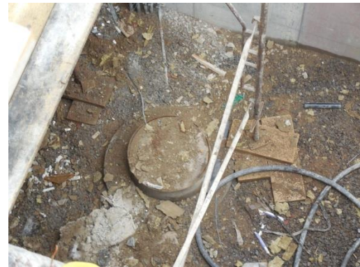
Figure 16: Sump Pump Well (Courtesy Jeremy Feath)
